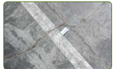
5. Concrete cracks by shrinkage or loads. Adding steel fibres not only works on temperature and shrinkage control, but increases the load bearing capacity.
